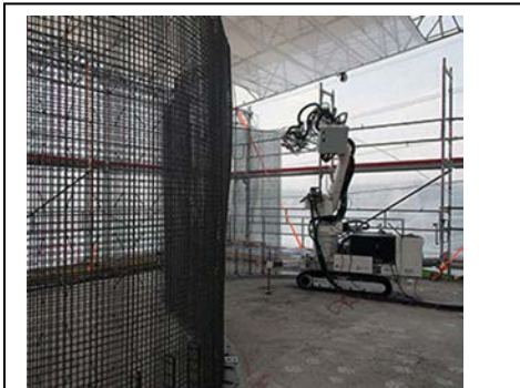
The mesh mold wall is built using the in situ Fabricator. Image: NCCR Digital Fabrication
